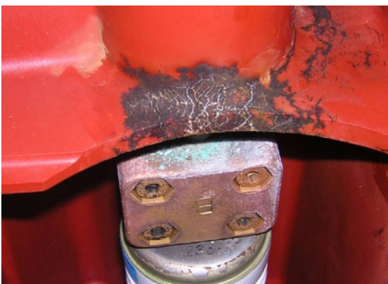
Figure 3: Tracking (surface) discharge damage. Image by Manning22S , own work, CC BY-SA 3.0
